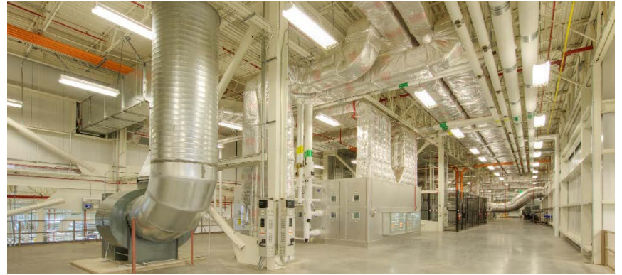
Efficient mechanical systems and lighting controls promote energy conservation
